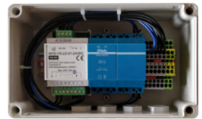
LIFT control box
